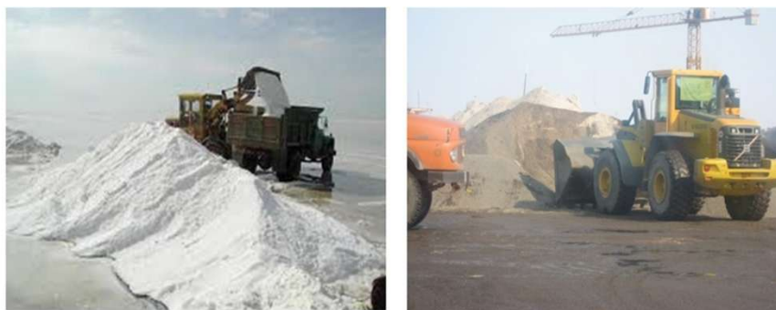
Fig 1. A view of salt and sand piling in order to prevent formation of ice and snow layer in winter
