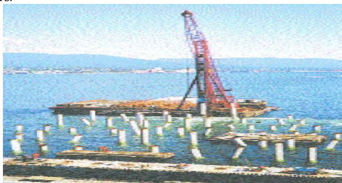
Figure 1 - View of a bubble curtain in place of berthing the ship in Vancouver of Canada to reduce noise pollution [2].
