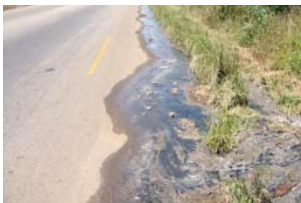
Fig 4. Sewage effluent from a burst pipe observed during sampling time.
