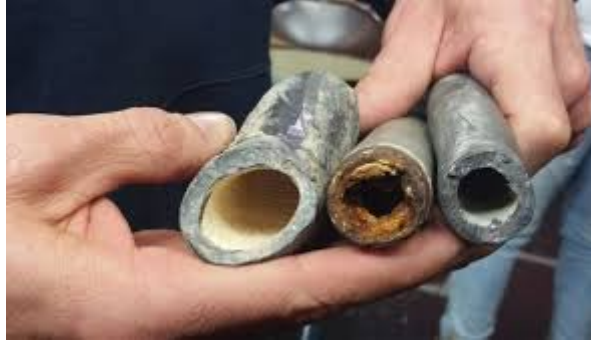
Fig. 2 Different Types of Corrosions in Drinking Water Pipes (Source – Google Images)
